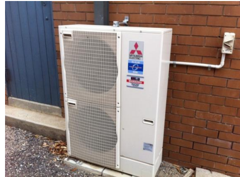
Air Conditioning Unit
